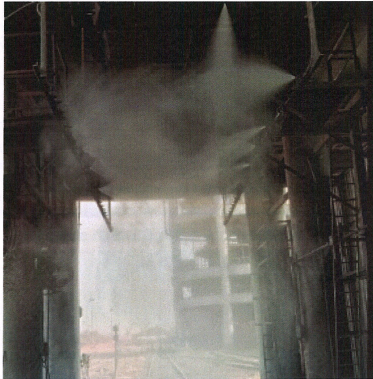
Mist System in hoppers
