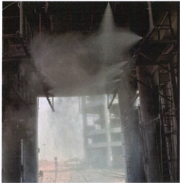
Mist System in hoppers
